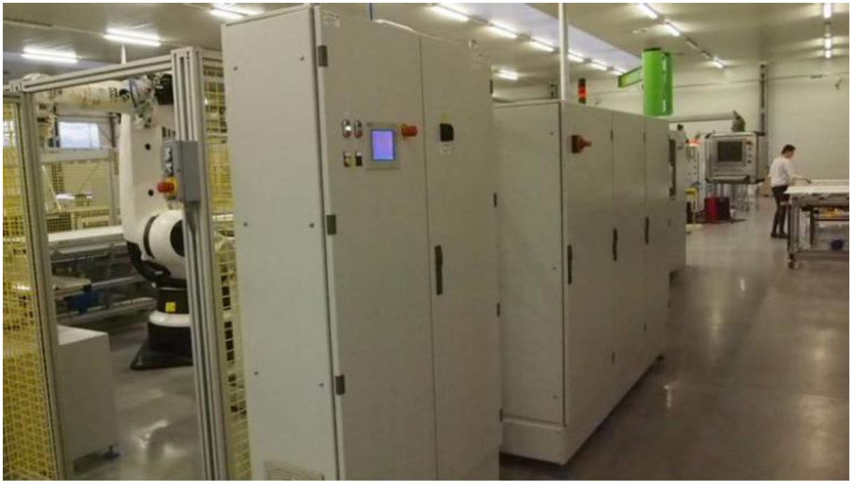
Control cabinets of Stringer
