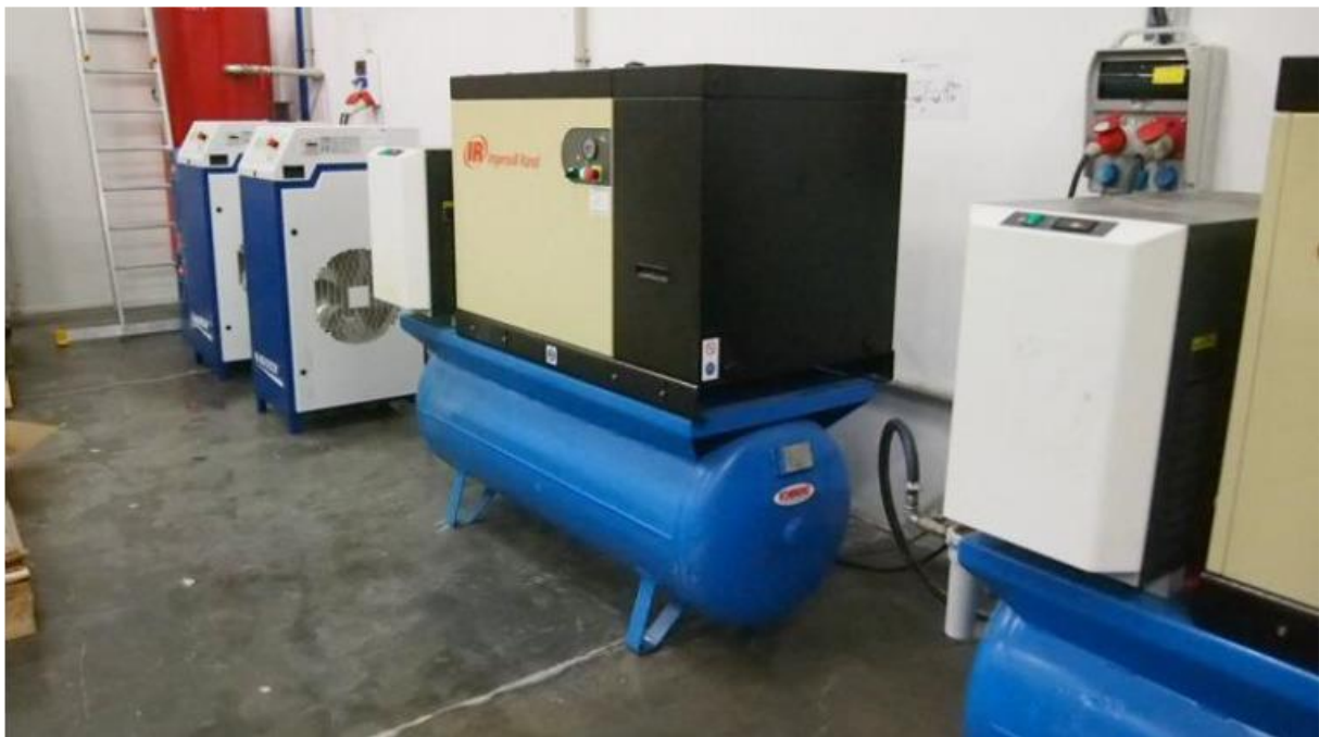
Compressed air station
